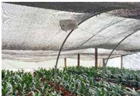
A fan heater used to warm the shade house.
